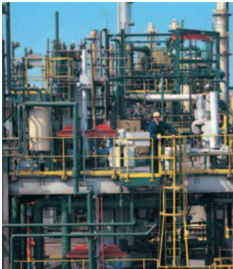
Frost protection of process lines
